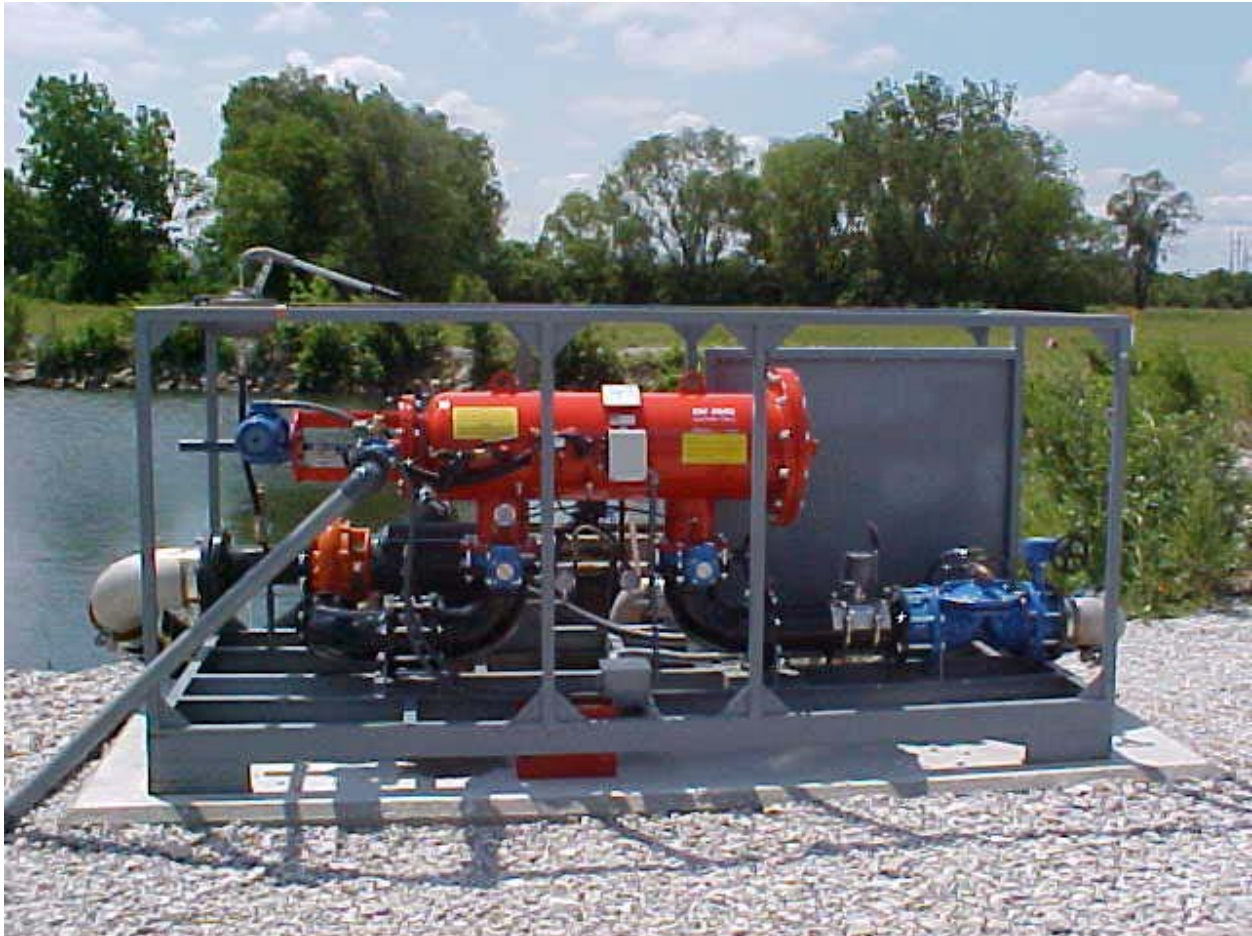
Figure 2 - Stormwater Treatment System (Back View)
